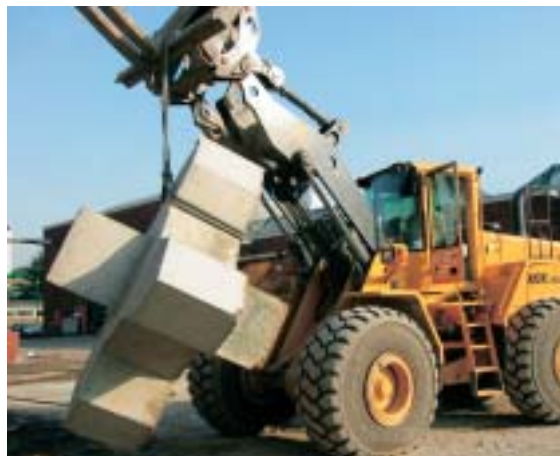
Figure 17. Handling the Xbloc® with a sling around the nose was the most suitable technique for placement.
